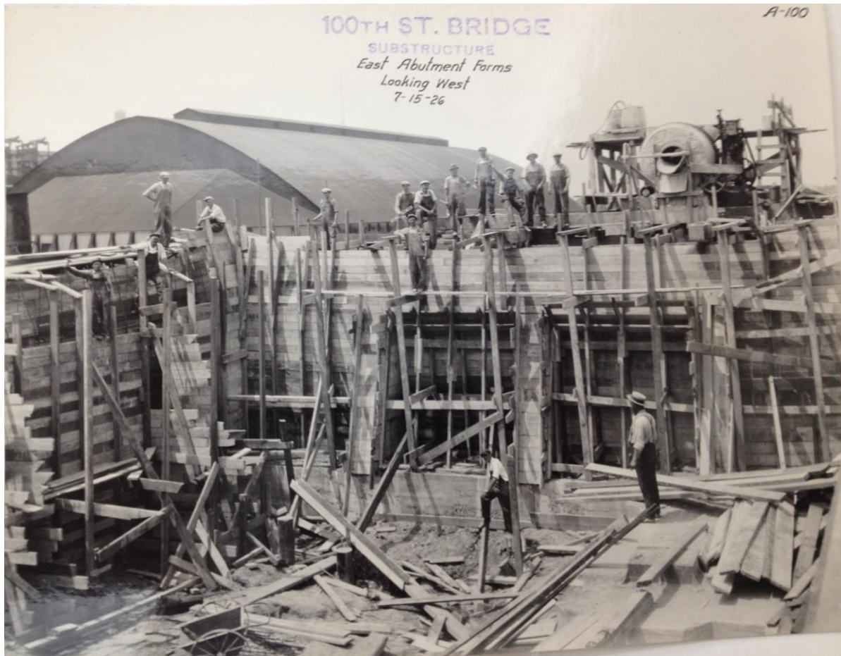
100 th Street Bridge substructure under construction looking west, July 15, 1926. Department of Public Works Photo Collection, 1860-1948, Chicago History Museum.
