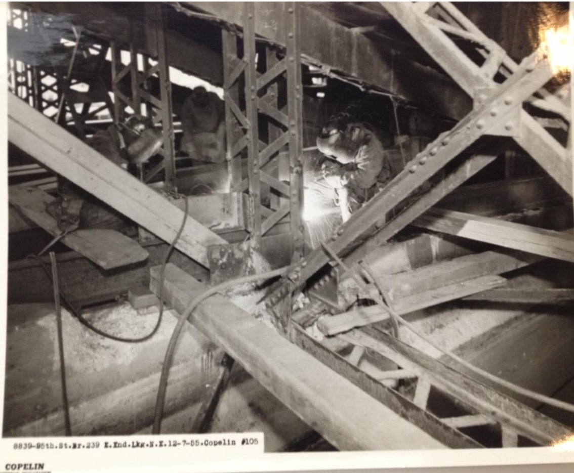
95 th Street Bridge, 1955. Photographer: Copelin. Department of Public Works Photo Collection, 1860-1948, Chicago History Museum.
