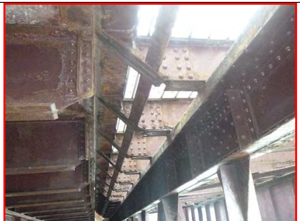
42. Section loss along a stringer in Span 3, looking southeast.
