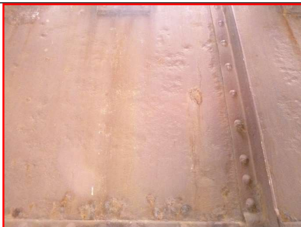
57. Typical floorbeam pitting, looking east.
