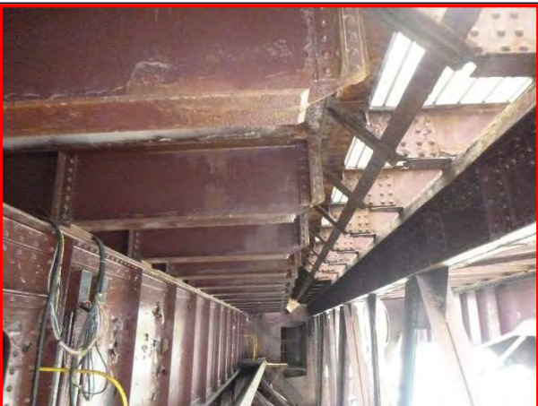
40. Stringer ends at east rear break, looking north.
