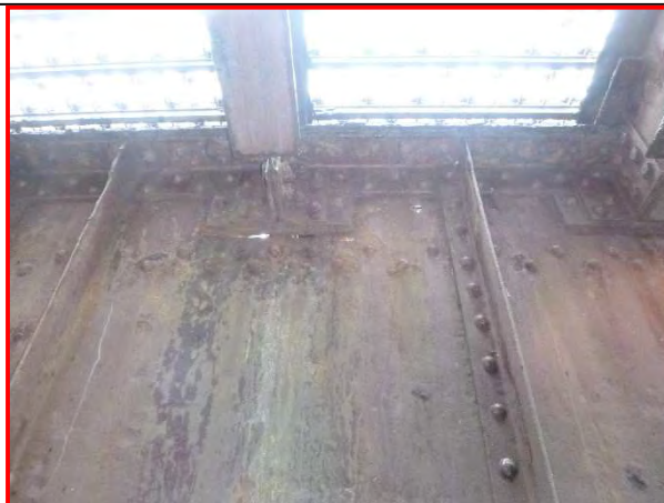
59. Typical corrosion hole near stringer connection, looking northwest.
