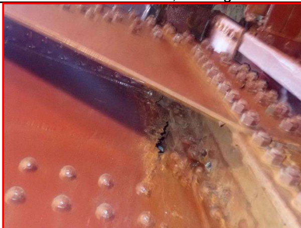
61. Southwest truss rear arm crack/corrosion hole, looking east.
