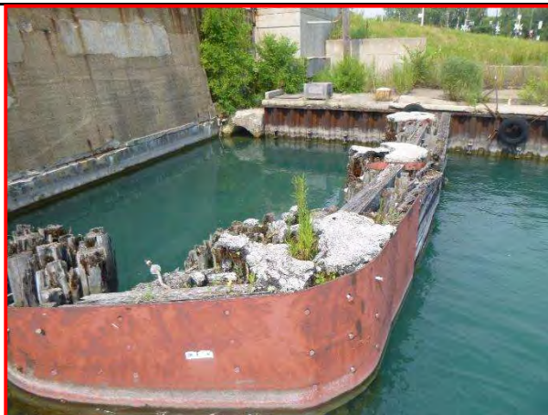
81. Typical condition of timber pile and steel plate protection system, looking north.
