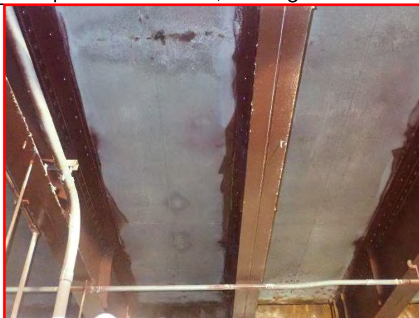
20. Typical transverse cracks in underside of fixed spans, looking south.
