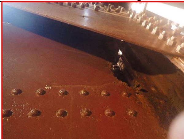
63. Northeast truss rear arm crack/corrosion hole, looking southwest
