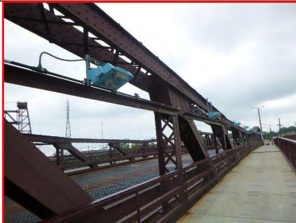
68. Lights attached to the truss, looking south.
