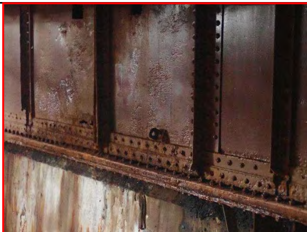
40. Hole in bottom of web in northwest longitudinal girder, looking southwest.
