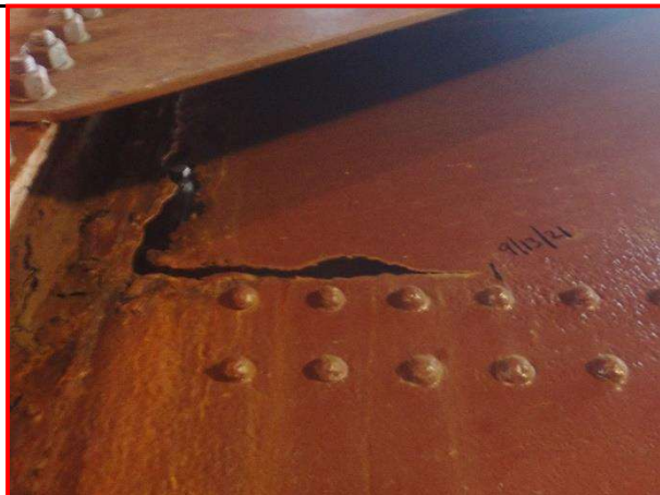
62. Southwest truss rear arm crack/corrosion hole, looking west.
