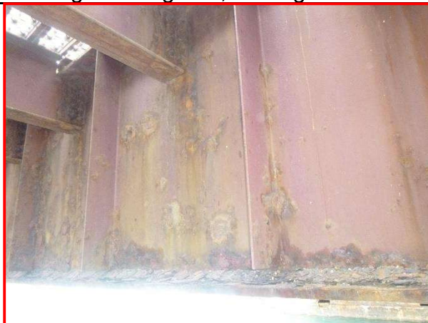
41. Typical moveable span floorbeam condition, looking north.
