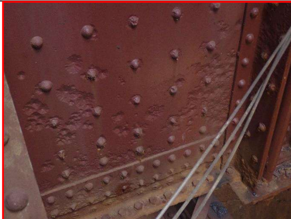
38. Moderate pitting to end bay of trunnion cross girder, looking south.
