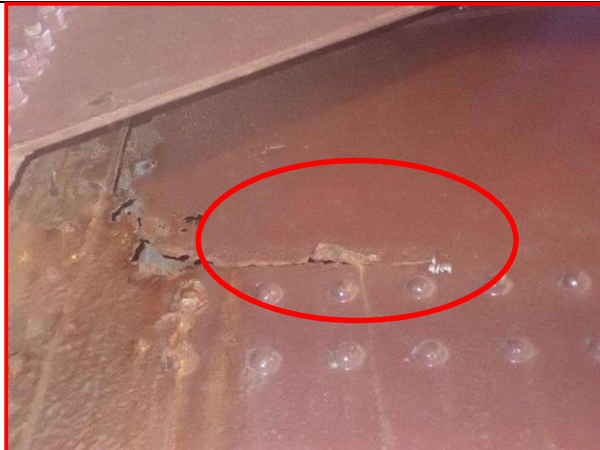
60. Southeast truss rear arm crack/corrosion hole, looking west.
