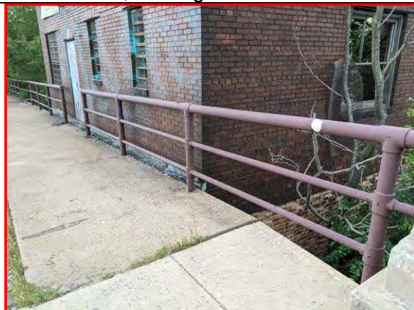
19. Guardrail at the southeast sidewalk, looking southeast
