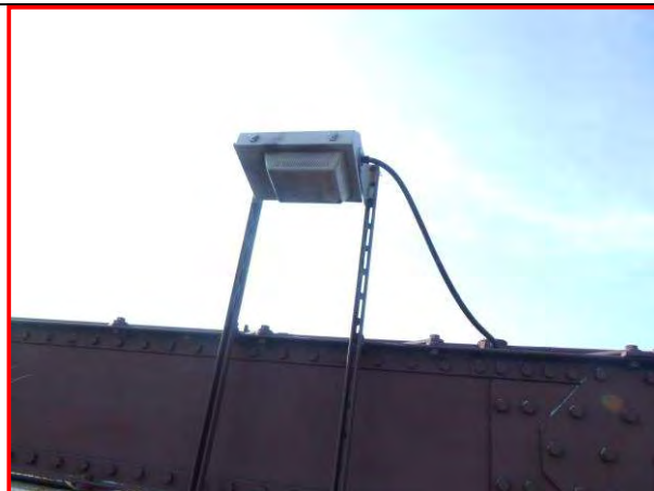
54. Lights and conduit attached to the top truss, looking south
