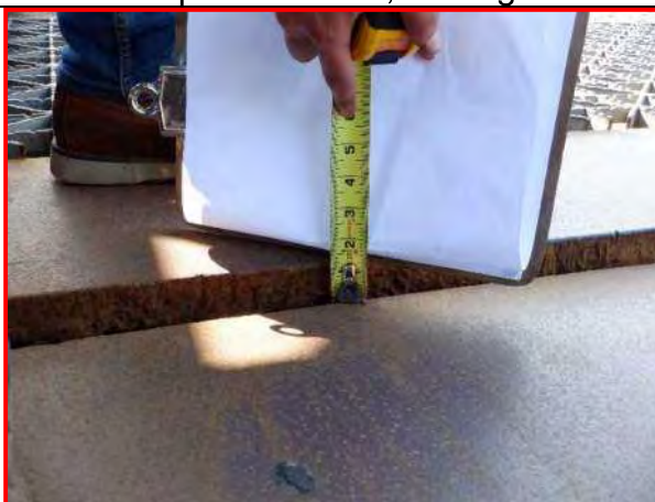
20. Vertical differential at center break, looking west
