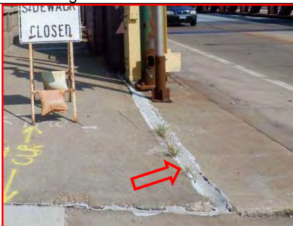
23. Northwest sidewalk joint, looking east
