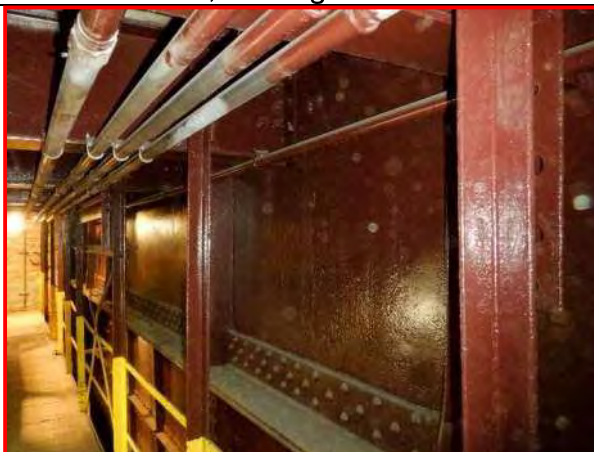
79. Span 1 conduits, looking south
