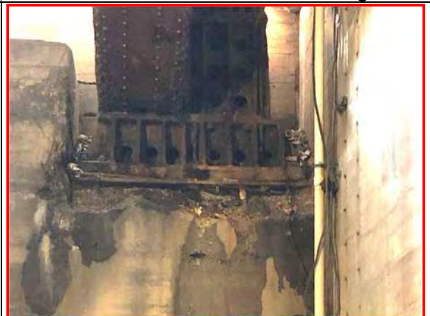
84. West River Pier inside face at the south trunnion girder bearing, looking east
