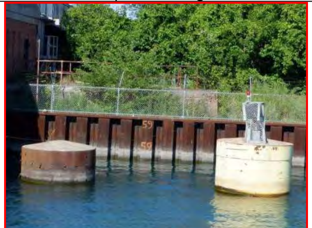
94. Light cage on the northwest dolphin, looking west
