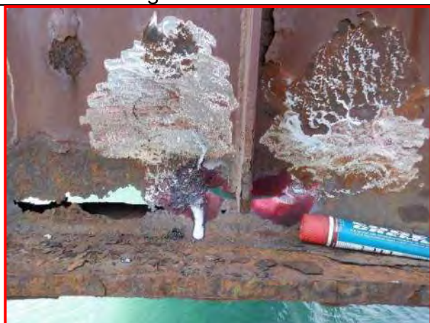
53. FB 0-0W crack, looking west
