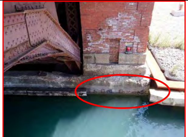
92. Timber fenders missing on East River Pier, looking east
