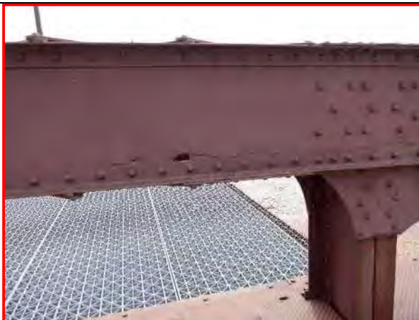
67. Top chord corrosion hole, looking south
